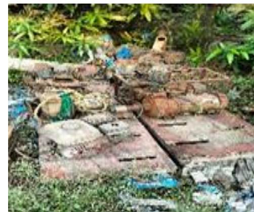
Dewatering Pumps /submersible
