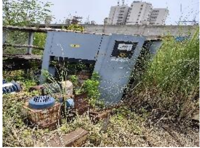
Damaged air compressor
