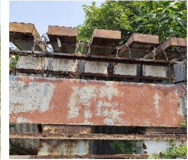
Cut out panel unit Damage
