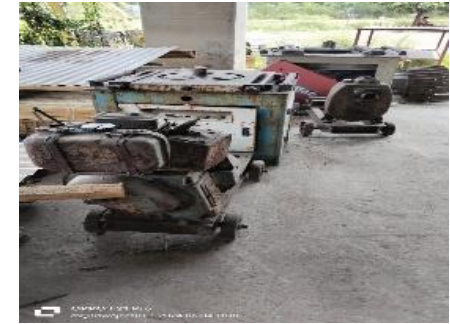
Diesel pump (7.5 kv DG)
